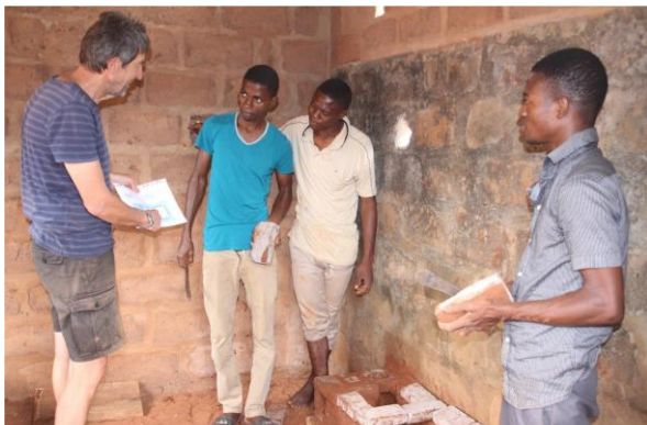
The plan is checked carefully before starting construction: Frank, Jean-Philippe, Joseph and Didier
